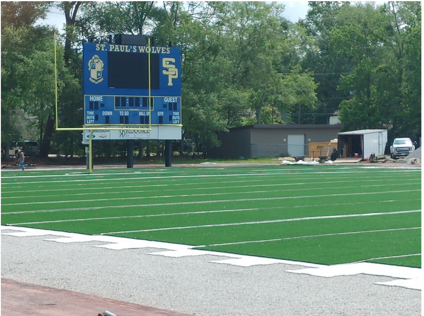
The new turf is laid over the gravel and impact pad base on the stadium field.
