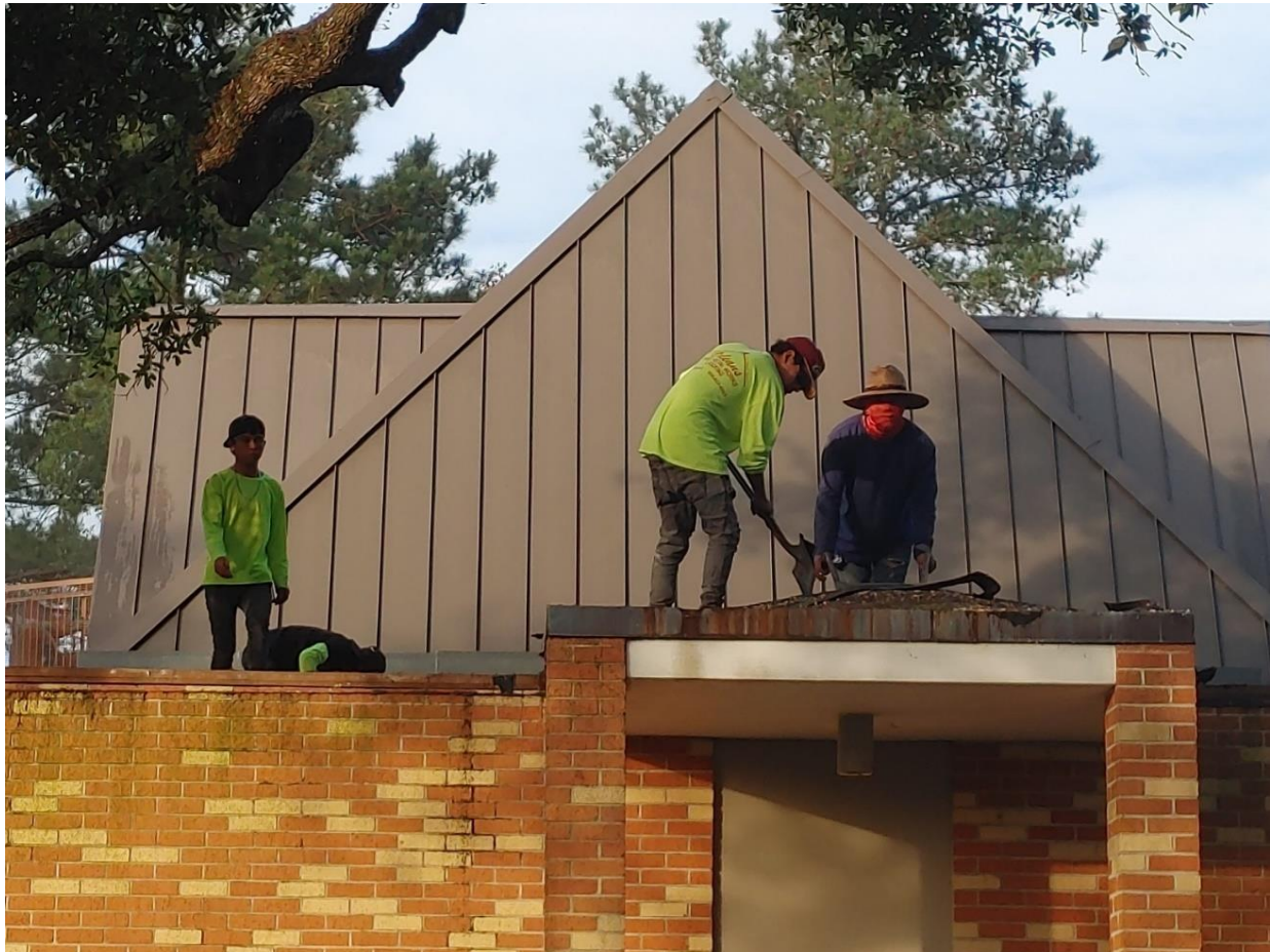
Above: Workers remove the old chapel roof to prepare the surface for the new roof.
