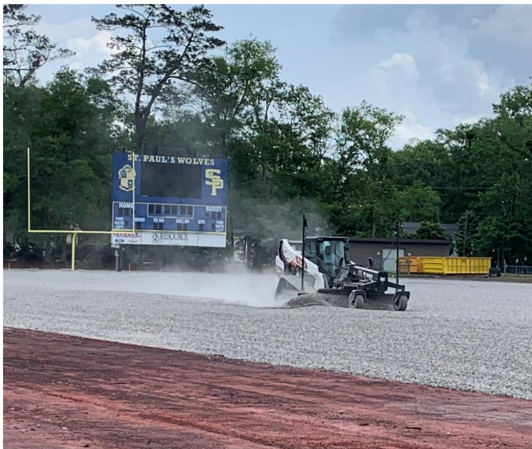
Left: Leveling of the limestone subsurface is underway. Next up: laying the underlayment impact pad.
