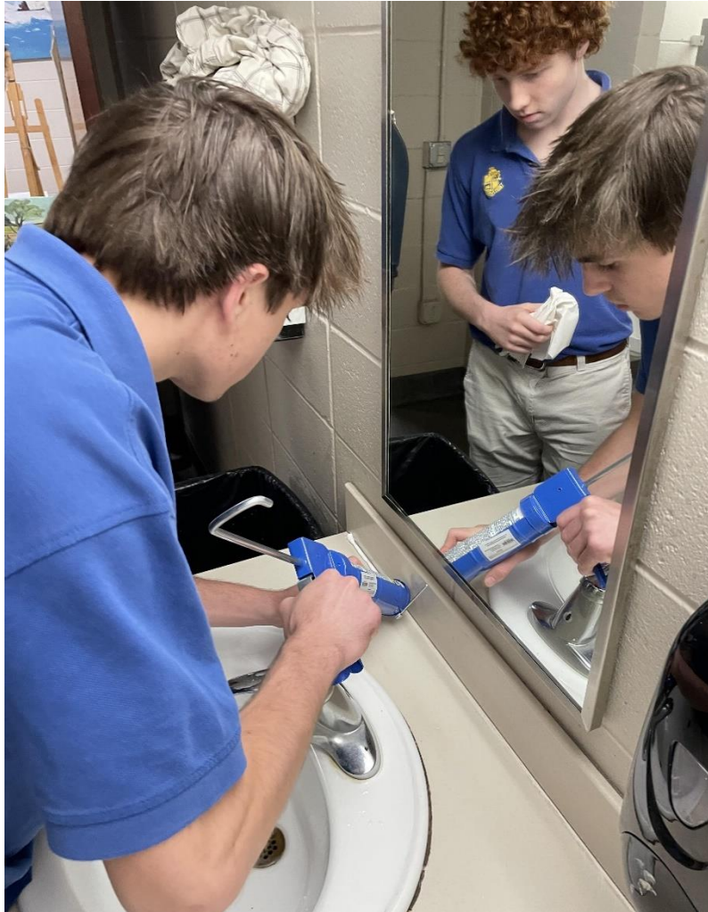
Left and Above: Members of the St. Paul's Fix It Club repair the caulk for the sinks and counter in a bathroom in LaSalle Hall. The students practiced with cardboard before putting their new skills to work to help improve their campus.
