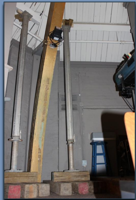
Damage to the theater was discovered after the initial assessment.
